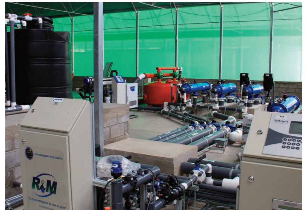
Water recycling system at Las Limas is state-of-the-art, providing both excellent crop irrigation and nutrition, and environmentally sound water management.
